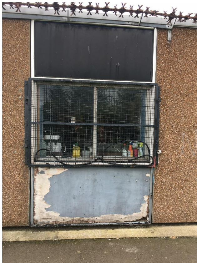
Example of a Condition 'D' (Bad) Community Centre External Wall (Building Element Level)- Clovenstone Community Centre
