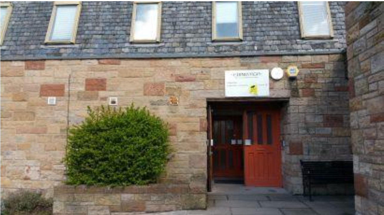
Example of a Condition 'B' (Satisfactory) Community Centre (Overall Building Level)- Craigentiny Community Centre
