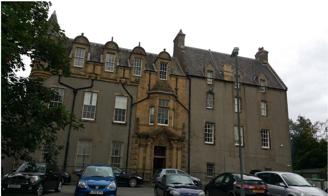
Example of a Condition 'C' (Poor) Community Centre (Overall Building Level)- Inch House Community Centre
