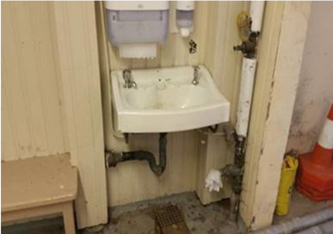
Example of a Condition 'D' (Bad) Community Centre Toilet (Building Element Level)- Castleview Community Centre
