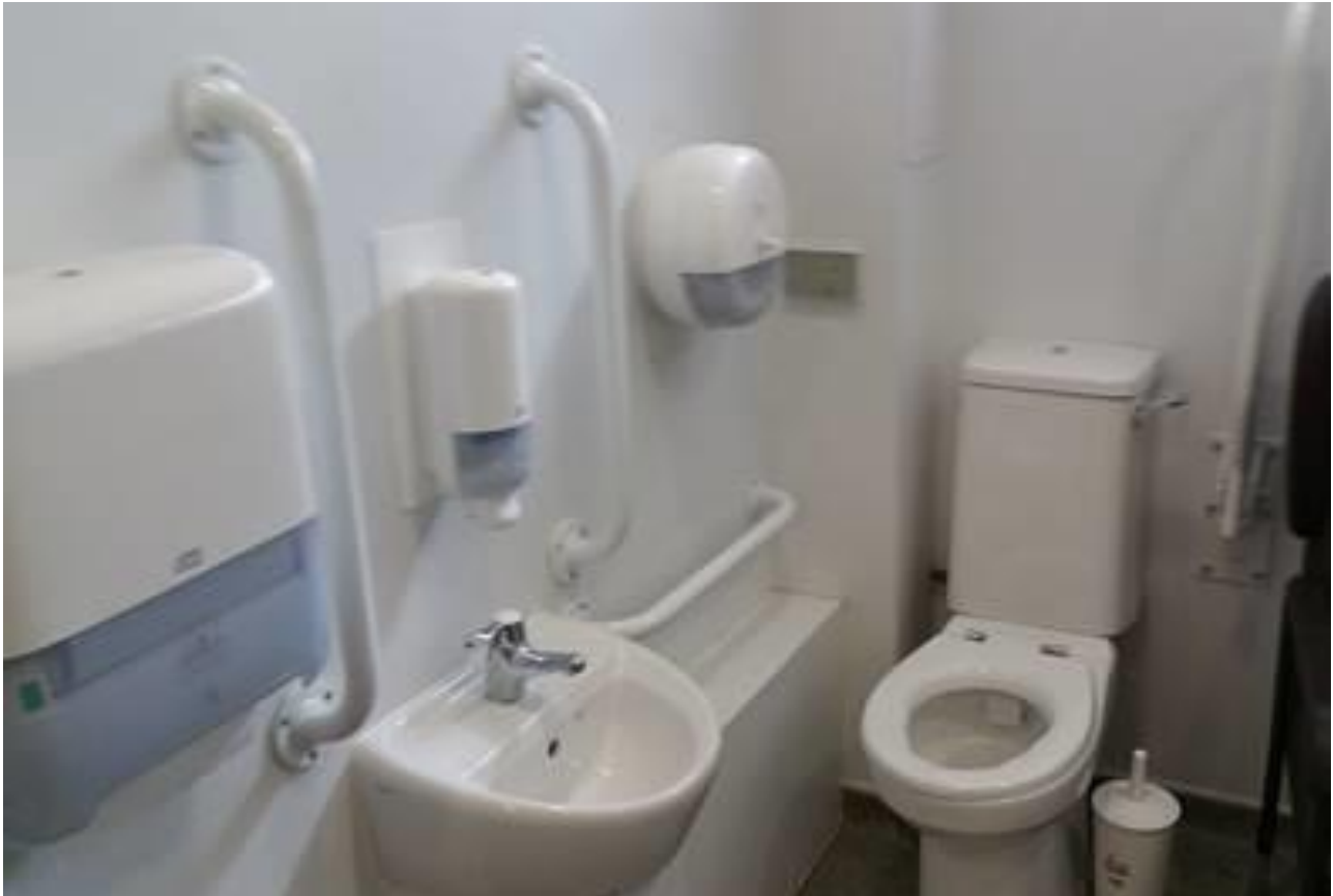
Example of a Condition 'A' (Good) Community Centre Toilet (Building Element Level)- Royston/Wardieburn Community Centre
